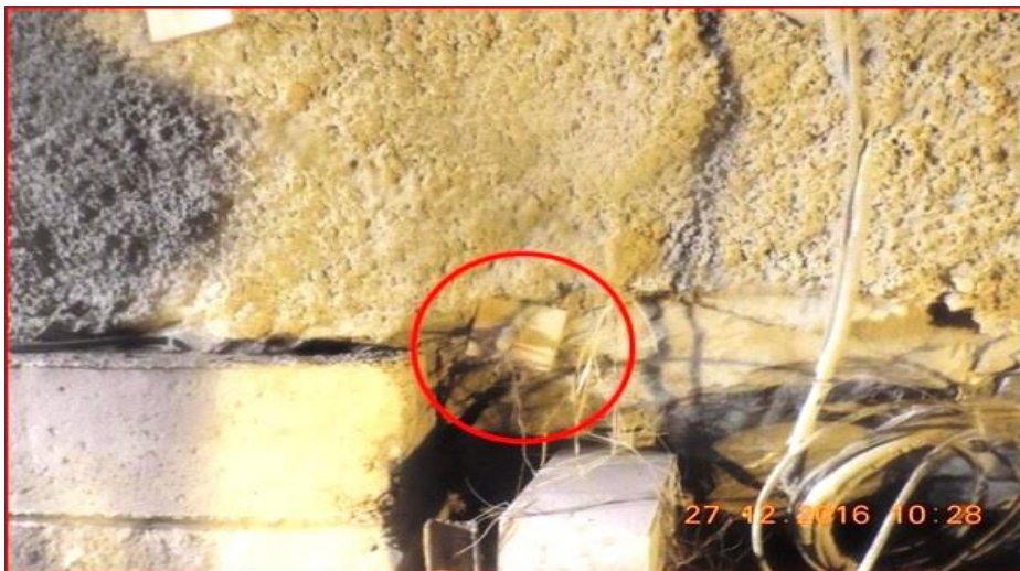
Figure 7 Bending in bearing plates of rock bolts (encircled in red)
