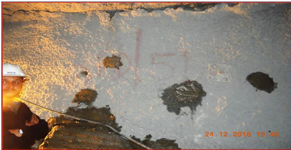
Figure 6 Rock bolt failures at RD 51.0 m
