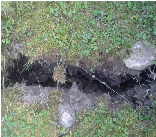
Photograph 2 Surface Cracks above the Cavity Zone
