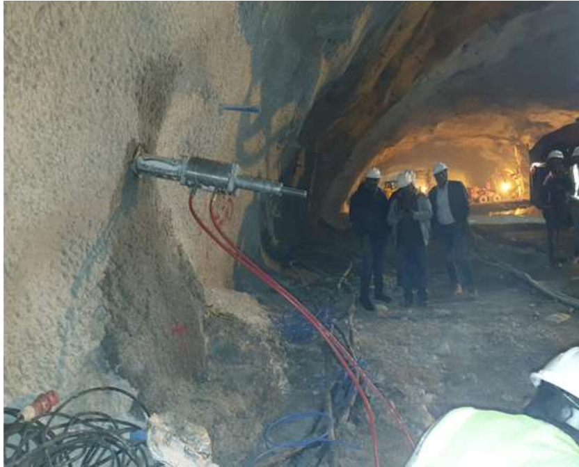
Picture 2 Showing Pull-out Testing Equipment & Experiment-2 (a,b) Pull-out at RD132m (R-8 hole, EL 1279, Right SPL- Stage-2 heading portion of PH cavern) in sheared & fractured weak rock mass–View from Top Adit to PH Crown towards Main Access Tunnel
