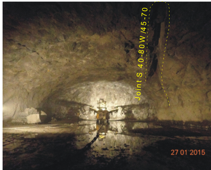
Figure 4 Open joint at the right crown of pump house
